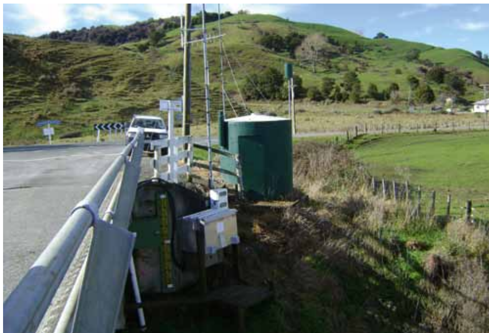
Above: Kanakanaia telemetry station, which records data on the Waipaoa River.
