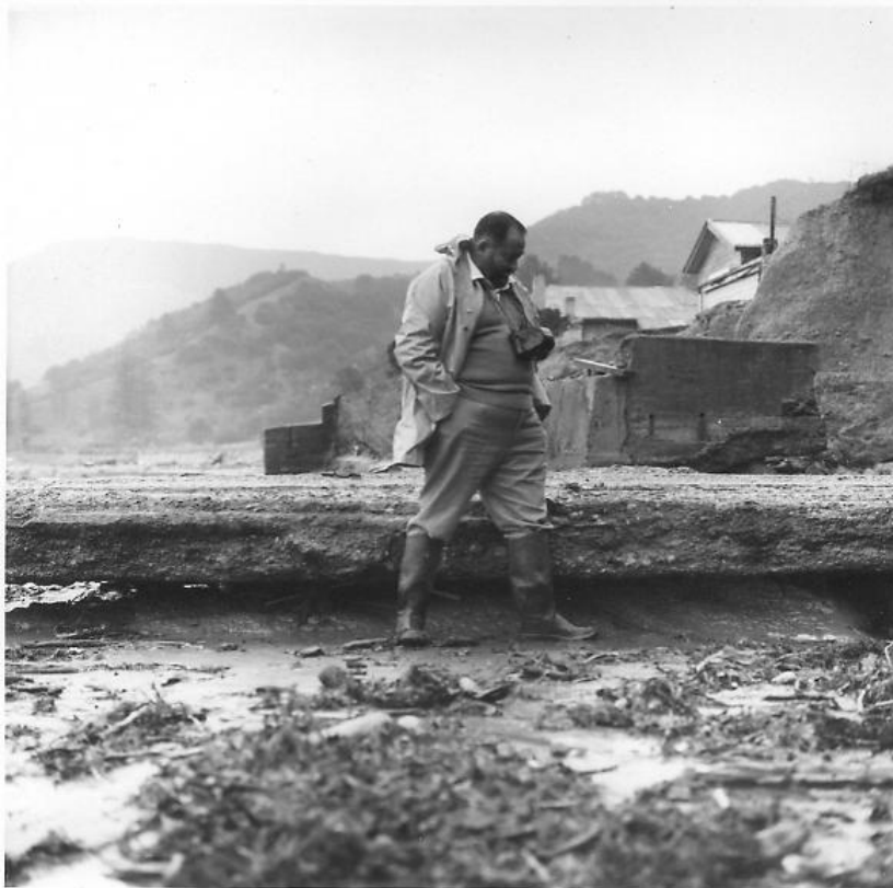
• Figure 4: Photos taken in July 2008 (top) and June 1980 (bottom) showing about 0.20m downcutting of the shore platform plane at Waima, northern Tokomaru Bay, over the last 28 years at 7-8mm/year beneath a section of concrete seawall destroyed earlier by the sea. Photos by JG Gibb.
