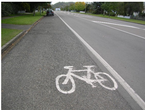
Smooth surface not carried into layby area, Ormond Road (Photo: Kim Smith)
