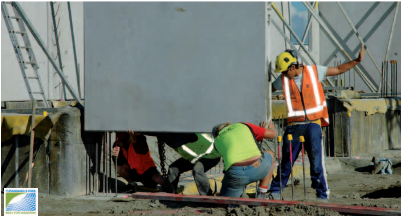
As a six-tonne panel is manoeuvred into position by crane, HEB Construction and Currie Construction workers help thread it over the starter bars that protrude from the footings. All the panels of the control room building have now been placed.
