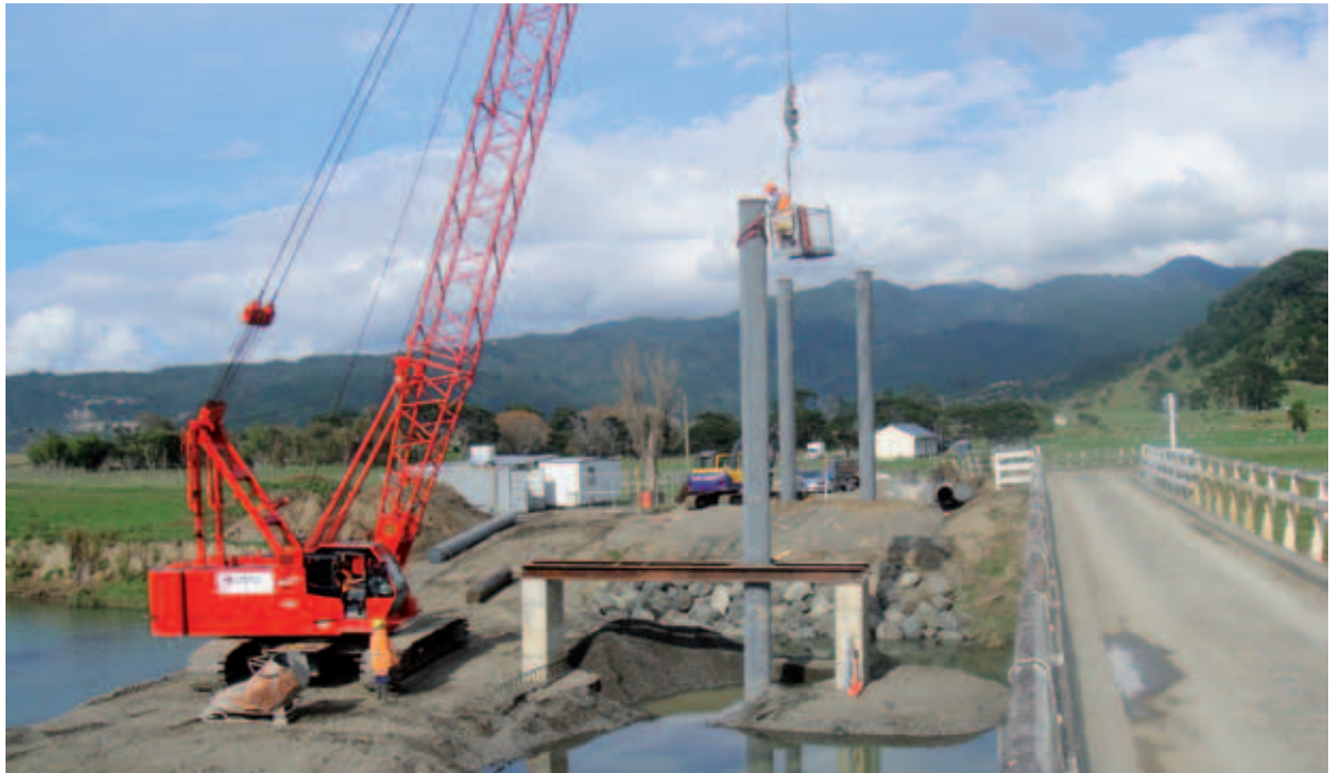
Piles are driven in for the new bridge across the Wharekahika River. Photo: Bob Elliott
