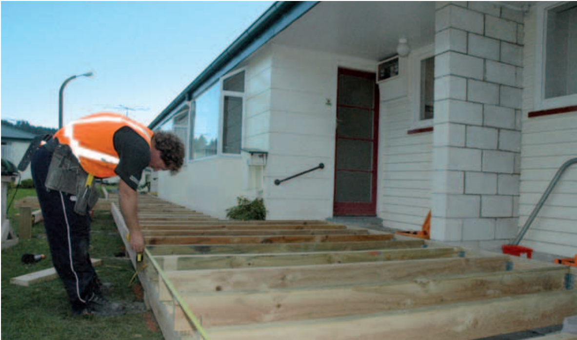
Watts & Hughes worker Chris Brown makes quick work of new decking at Council's Wildish Street units.
