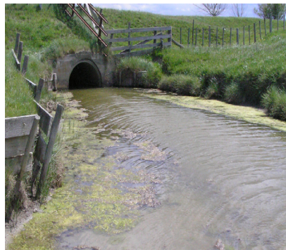
Inlet narrower than stream
