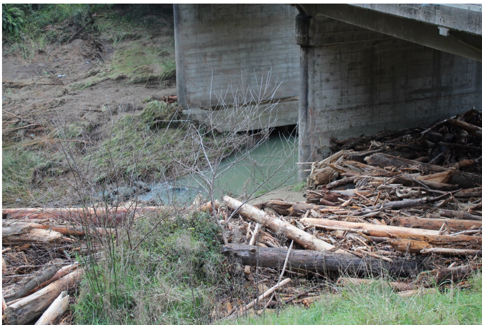
Damage to infrastructure – this is one of 5 SH2 bridges over the Maraetaha River – farm culverts, bridges and fences are also frequently affected by forestry slash mobilisation from slopes.
