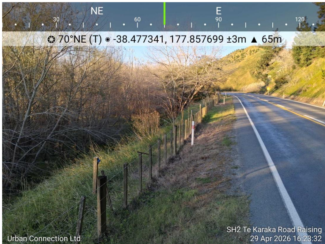
Figure 5.1-3: Drop-off into ditch / drain on SH2 (Site 1)
