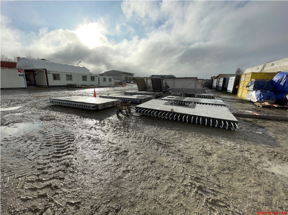
Precast panels ready for lifting into place for the tertiary flow splitter.
