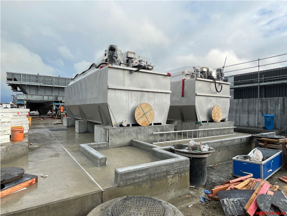
Tertiary filters in place on site.
