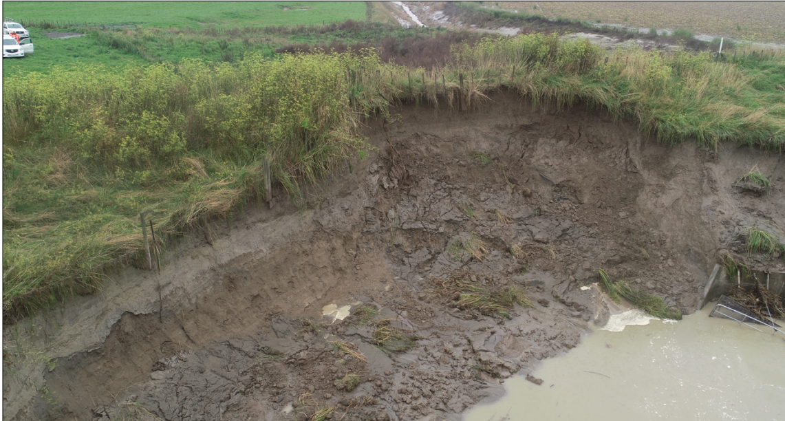
Photo 1 - Lavenham Road scour hole – Damage caused by Gabrielle.
