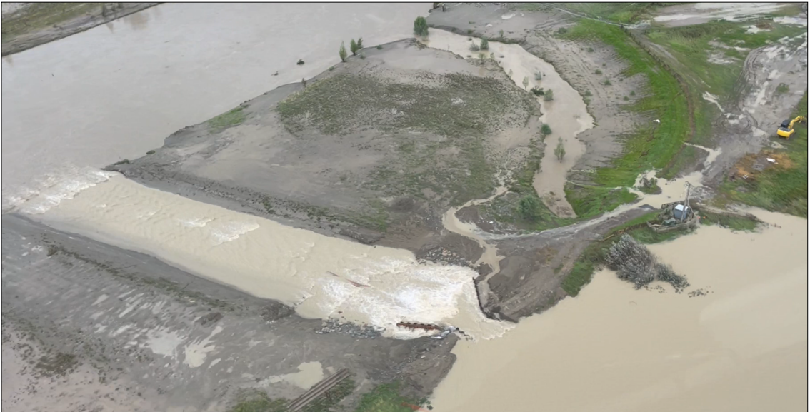
Photo 6 - Wi Pere Trust Spillway in operation during Gabrielle.
