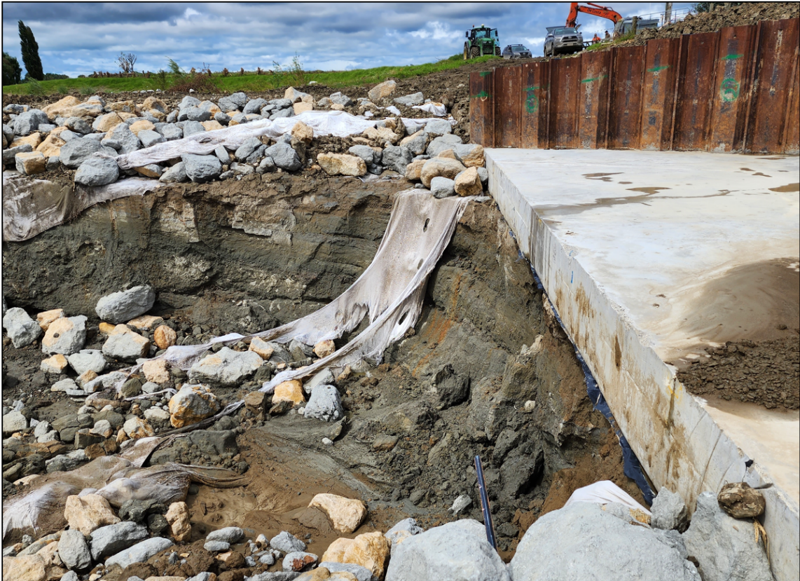
Photo 7 - Wi Pere Trust Spillway damage post Gabrielle.
