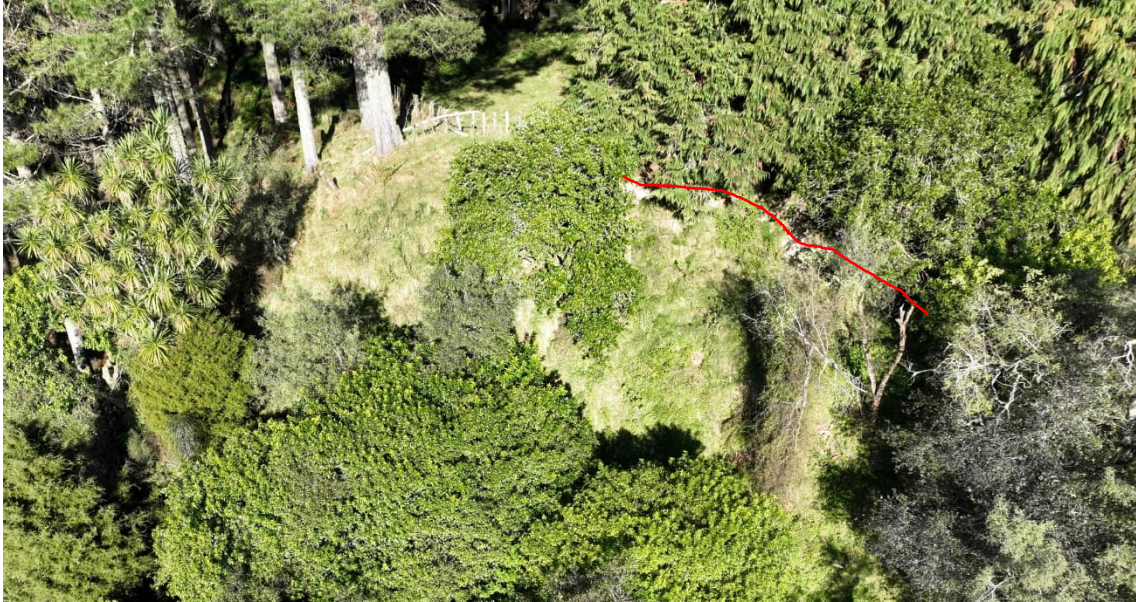
Figure 2: Tension cracking near the crest of Bluff 1 (marked by red line) exacerbated by recent low intensity rainfall.
