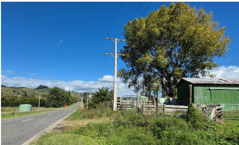
Figure 12 - Photo of the existing overhead power lines on Kanakanaia Road.
