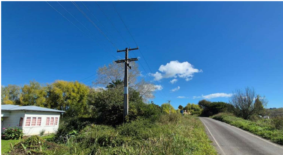
Figure 9 – Photo of existing overhead power lines on Rangatira Road.
