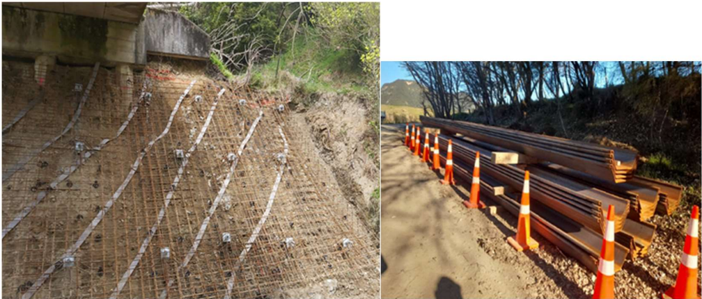
June 2018 -$1.5m - the last retaining wall structure was completed along Tauwhareparae road in September 2021.
