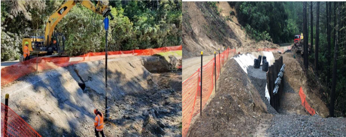
June 2020 -$11.1m - retaining wall structure again on Tauwhareparae Road was completed in October 2021.
