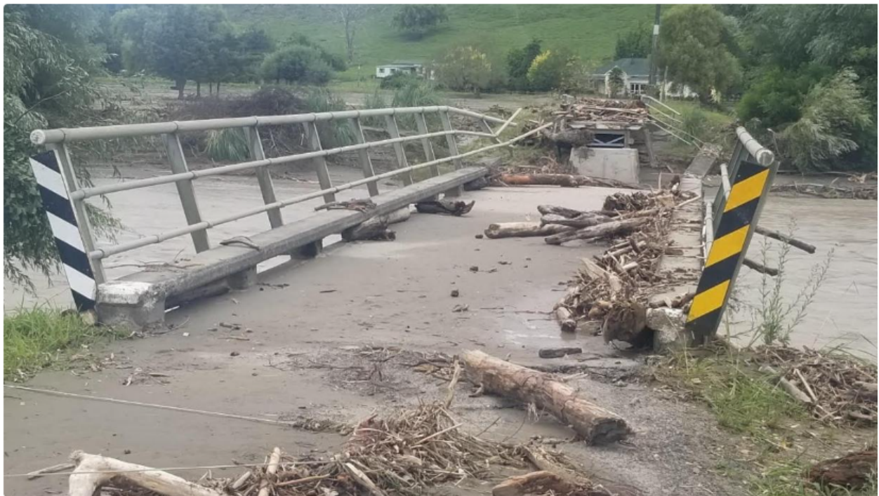
The old Mangatal Access Bridge across Waipaoa River was washed away during cyclone Gabrielle. Photo: Supplied / Not-For-Syndication
