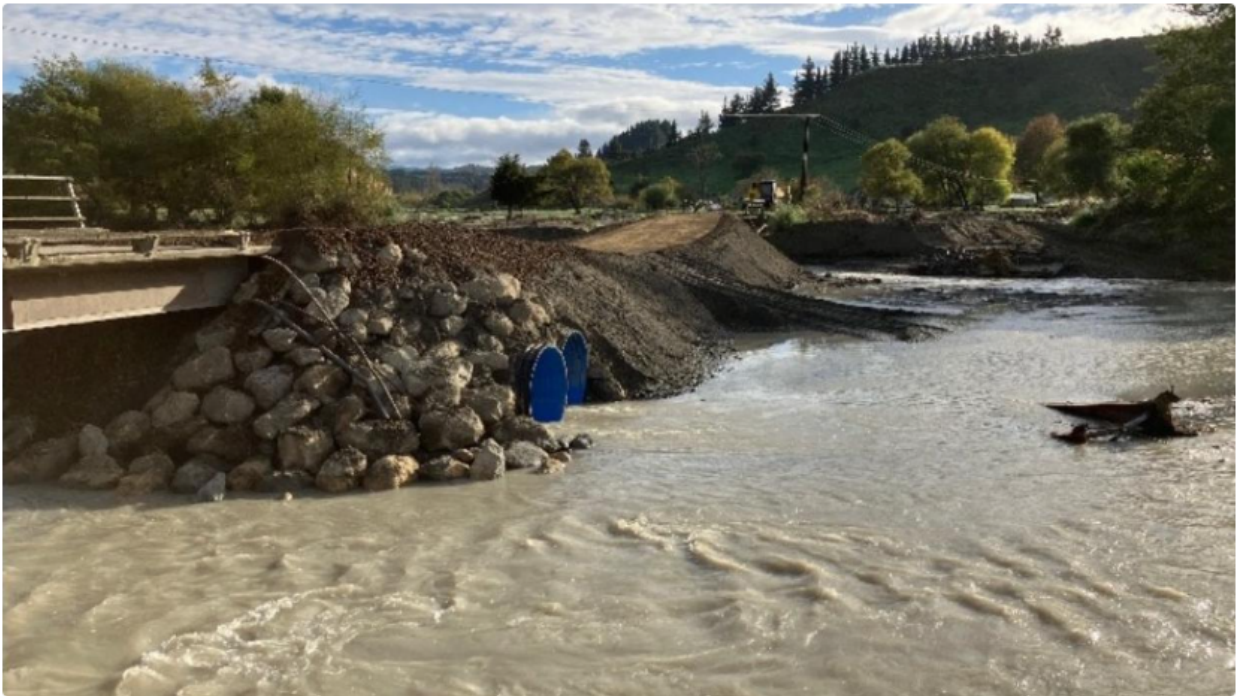
The temporary causeway on Te Kowhai Rd at Whatatutu in rural Gisborne has been washed away, less than a month after it opened. Photo: Supplied / Not-For-Syndication
