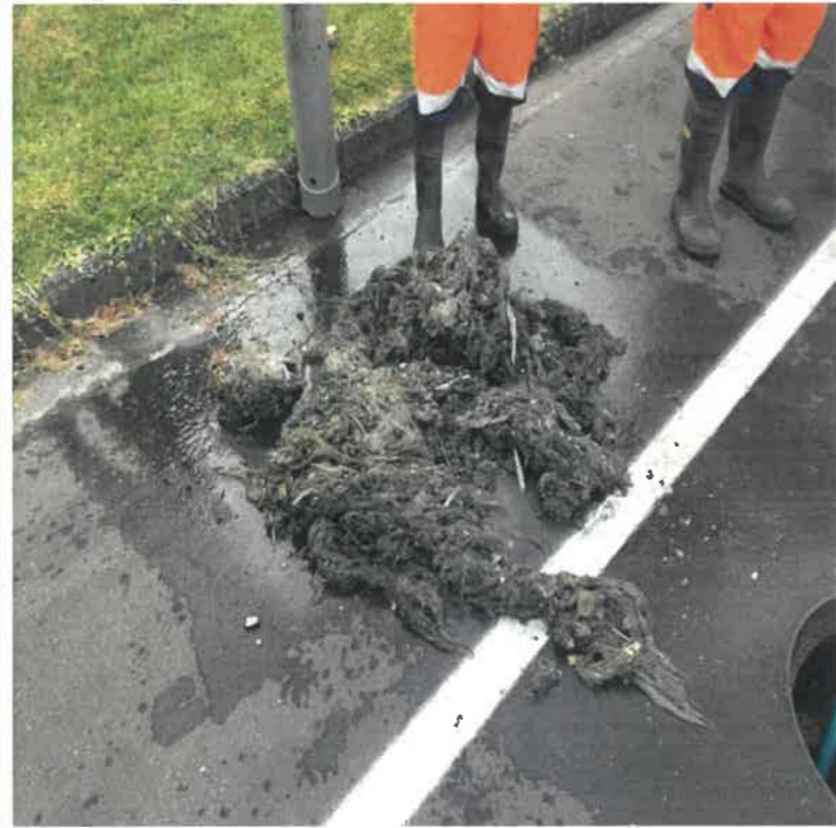
Sewer main in Stanley Road. Mainly composed of rags and wet wipes
