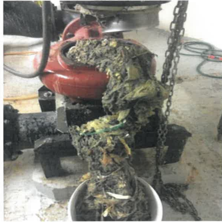
Childers Rd Pump Station caught in pump impellers. Rags, clothing, wet wipes, rope and more
