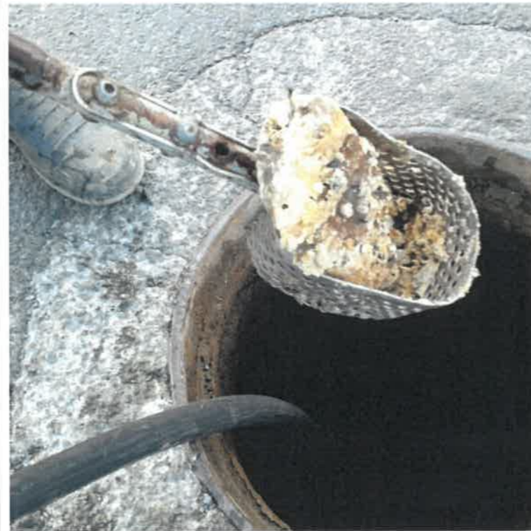
Ballance St. Solidified fat caught on rags of manhole
