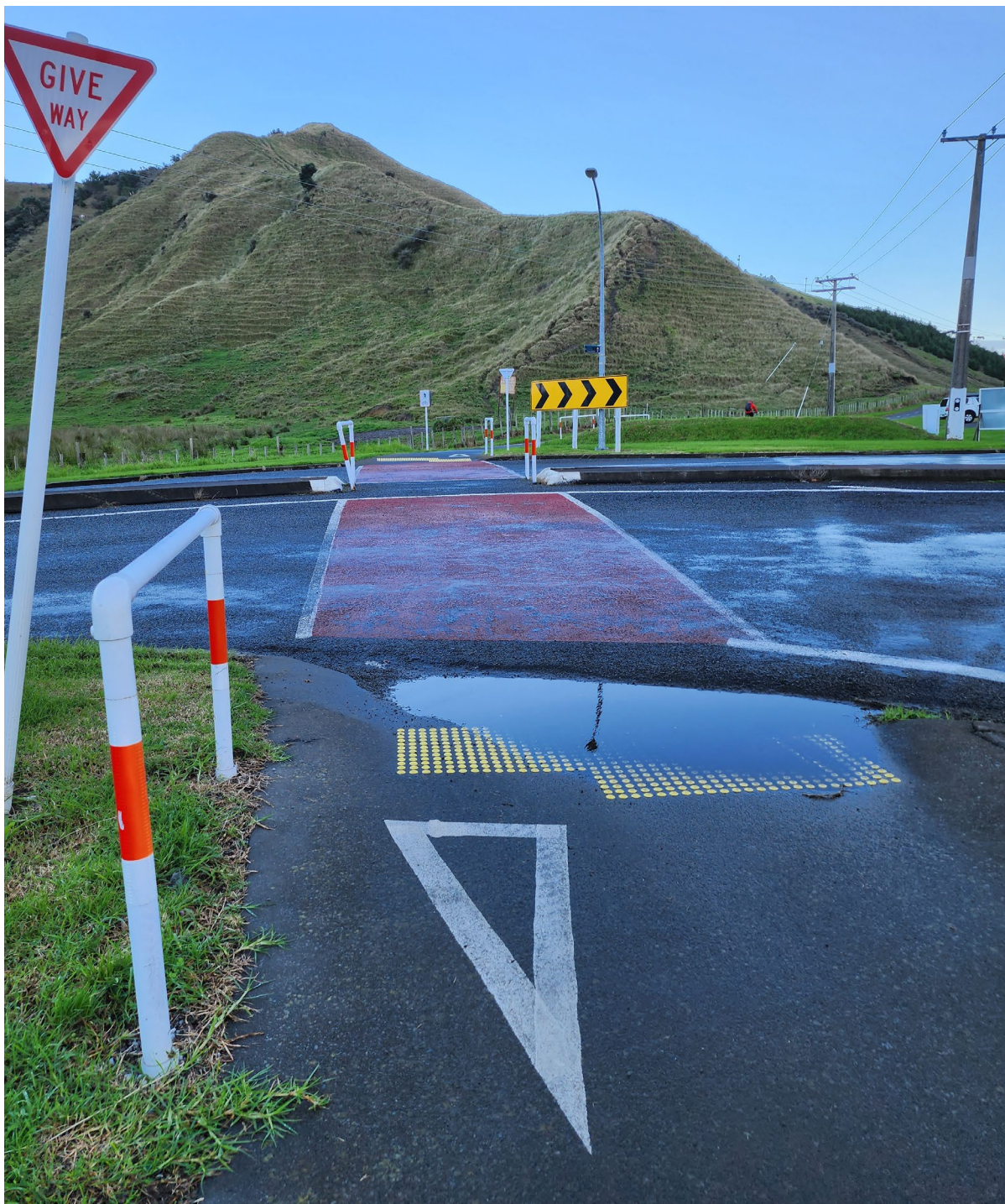
Figure 13 Example of poor drainage which covers tactile paving used by blind or partially sighted people
