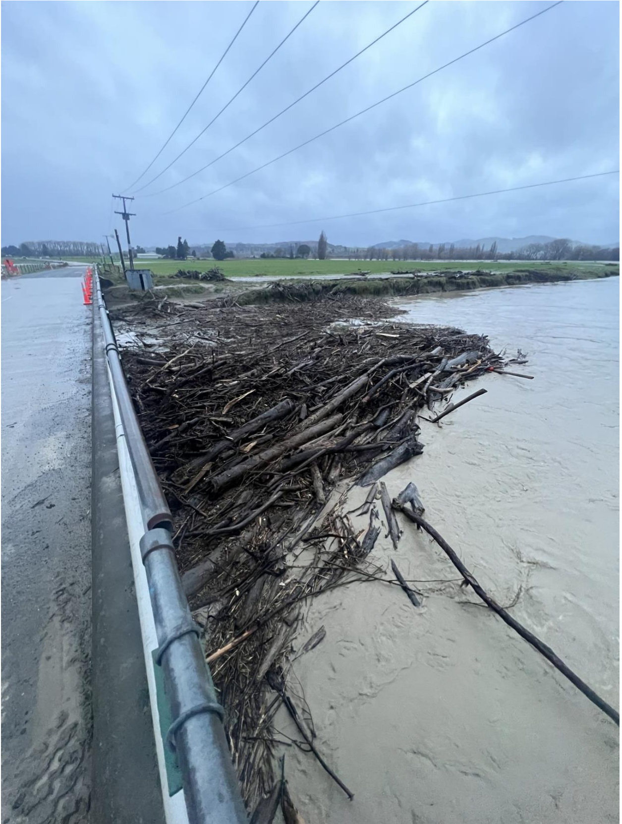
2. Debris raft against the Whatatutu Road bridge with the river still up. 23rd July 2023
