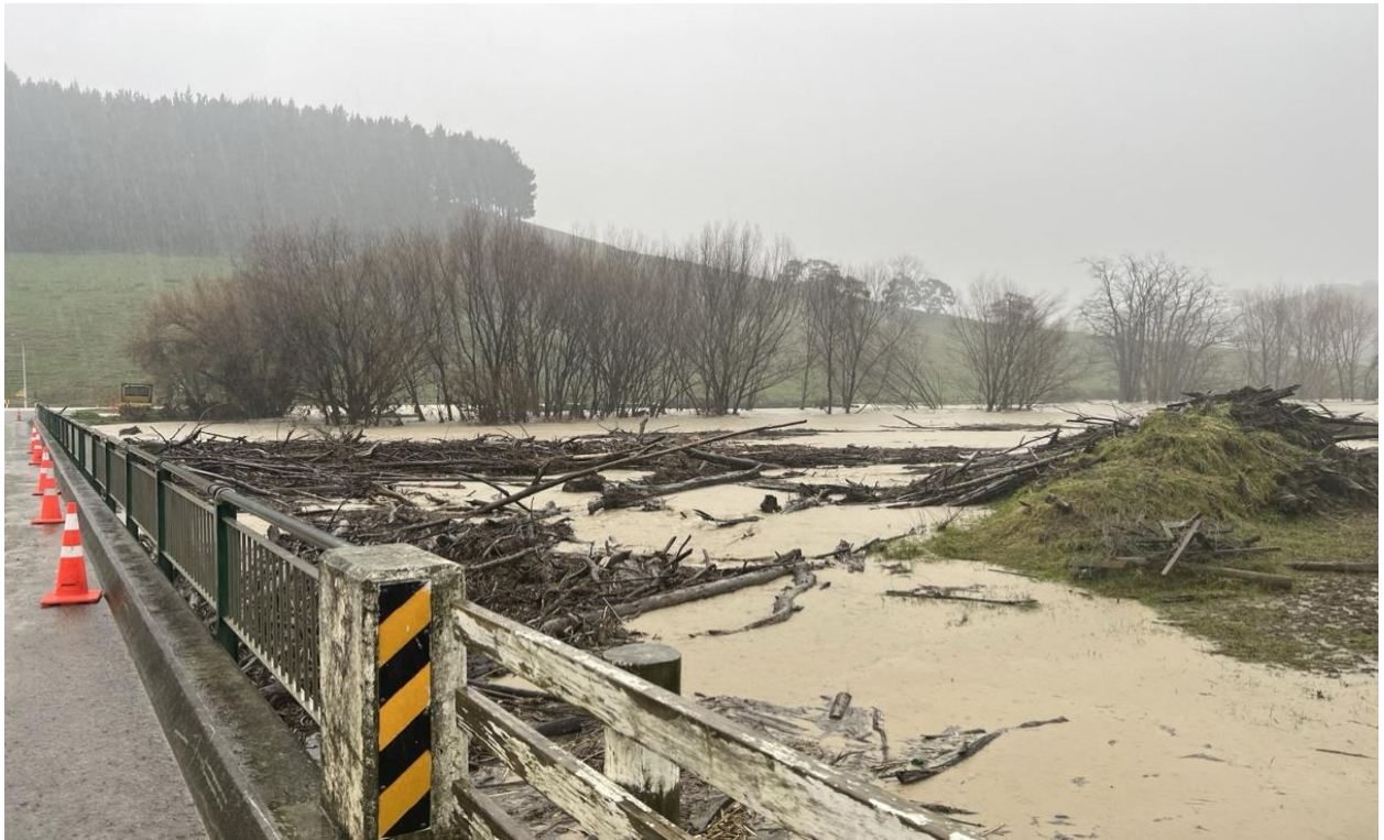
1. Whatatutu bridge, debris blockage. 22nd June 2023
