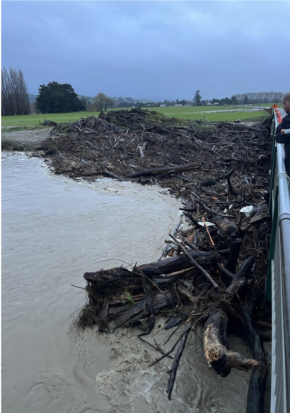
4. Wood debris piled against the bridge and bank as the water dropped. 23rd June 2023
