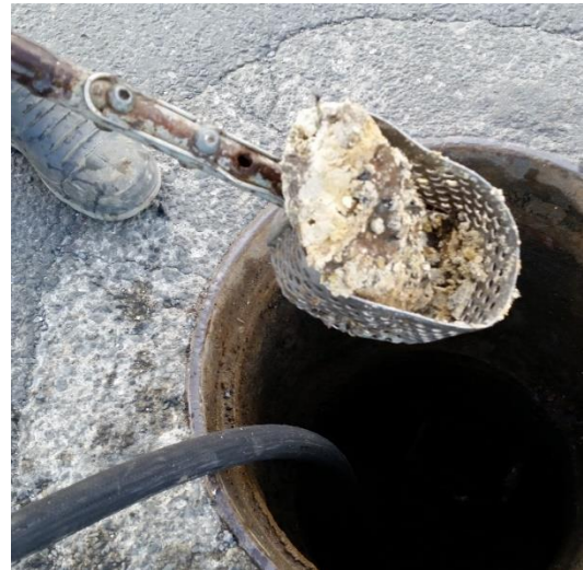
Ballance St. Solidified fat caught on rugs of manhole
