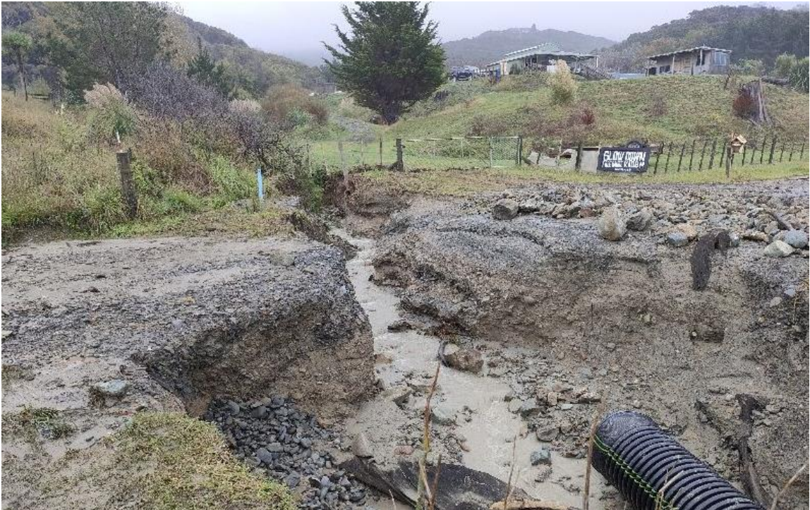
Below is damage on Waikawa Road at Waipiro Bay. The road is 4WD only and only open for residents.
