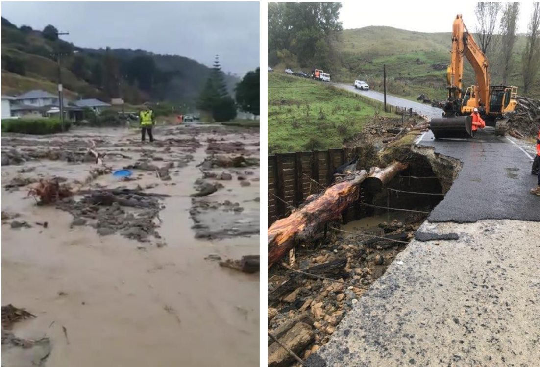
The below photo is on Puhunga Road which is now open again. The volume of water and the culvert possible becoming blocked has caused the flow to overtop the road and wash the road away. Existing culverts on the network are undersize for the intensity of the rain events we experienced.
