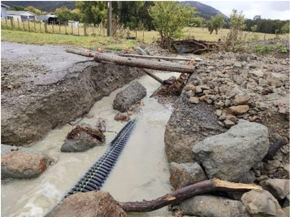
Below is the same type of culvert failure on Matahiia Road, the road is now open.
