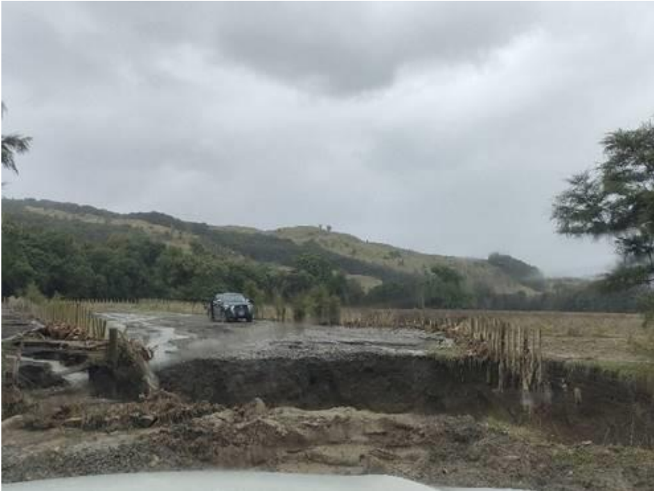
The below photo is another example of the same type of culvert failure on Mcllroy Road at Waipiro Bay. The road is now open again.
