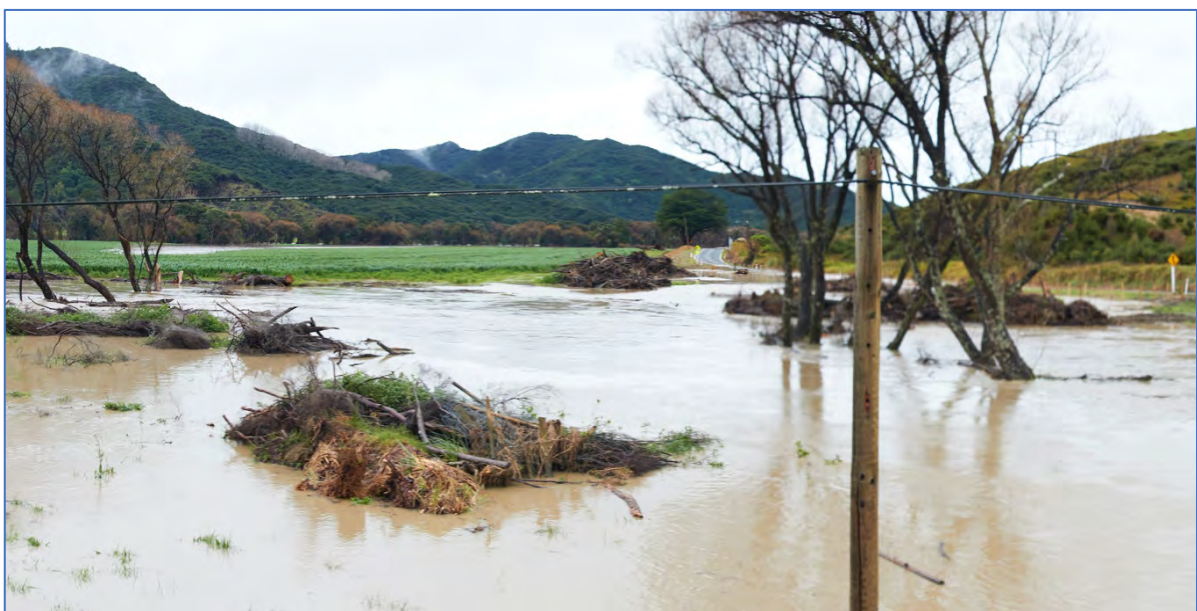
Figure Eleven. Willow piles being eroded upstream of State Highway 35 Bridge, Mahanga Stream. These were observed migrating to the Hikuwai River.
