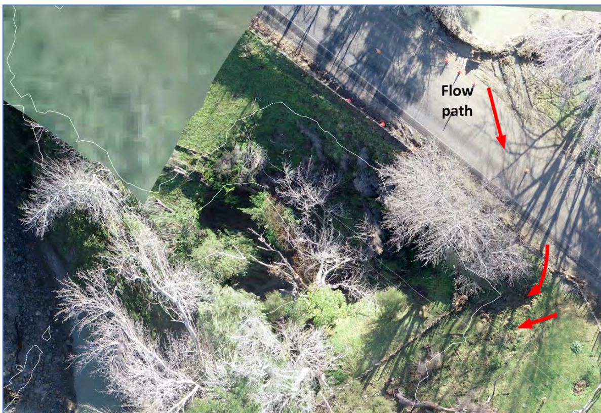
Figure Fifty One. drone footage of the blocked culvert on State Highway 35 showing the overland flow path to the creek downstream of the culvert.
