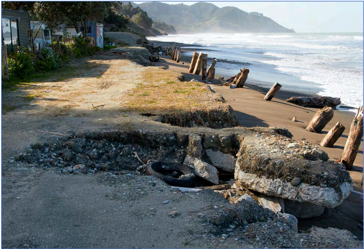
Figure Sixty Three. The extent of scouring and channelling of the road.
