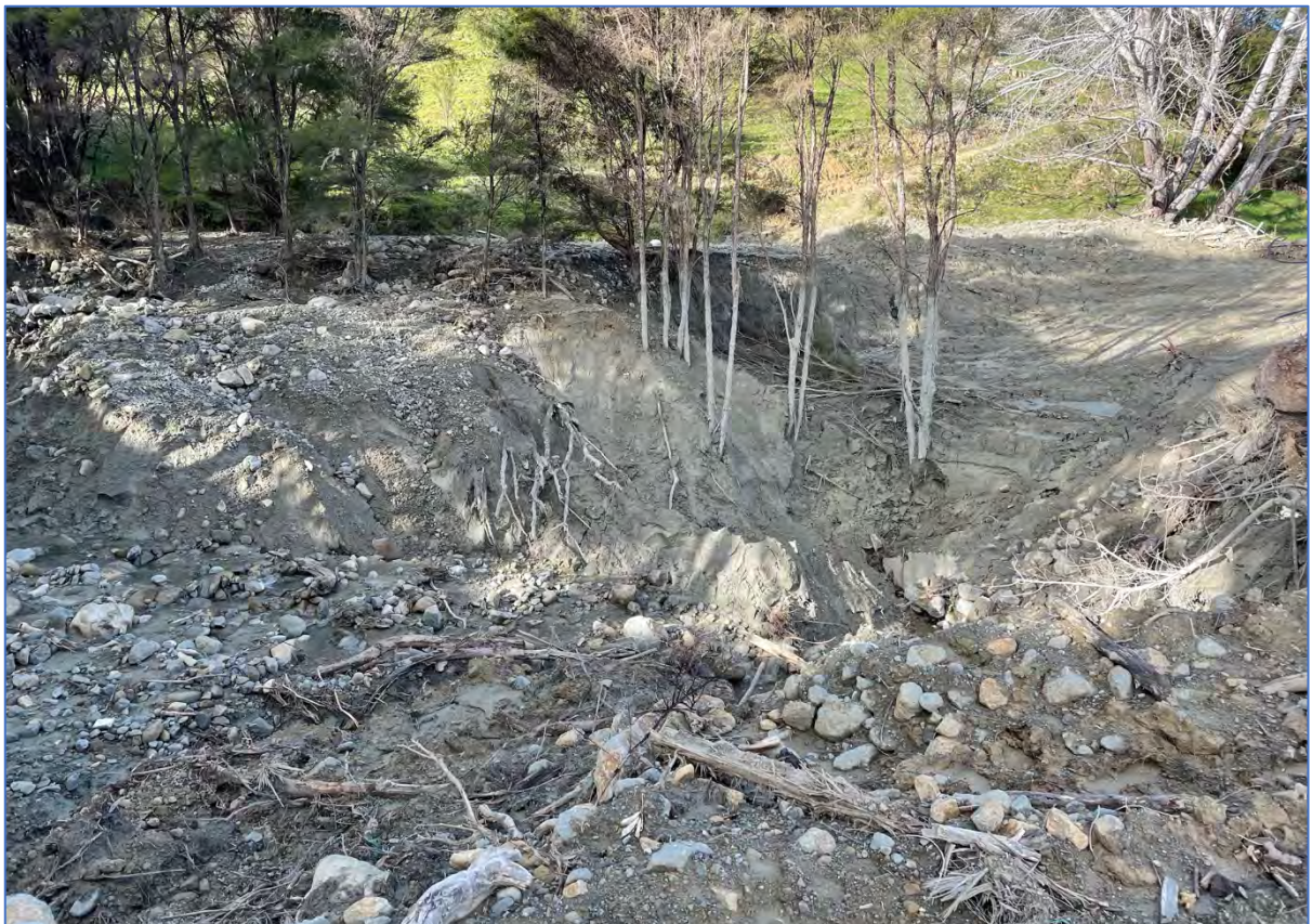
Figure Fifty Three. View of culvert on State Highway 35 north of Tokomaru Bay after clearing showing the considerable volume of debris remaining above the inlet.
