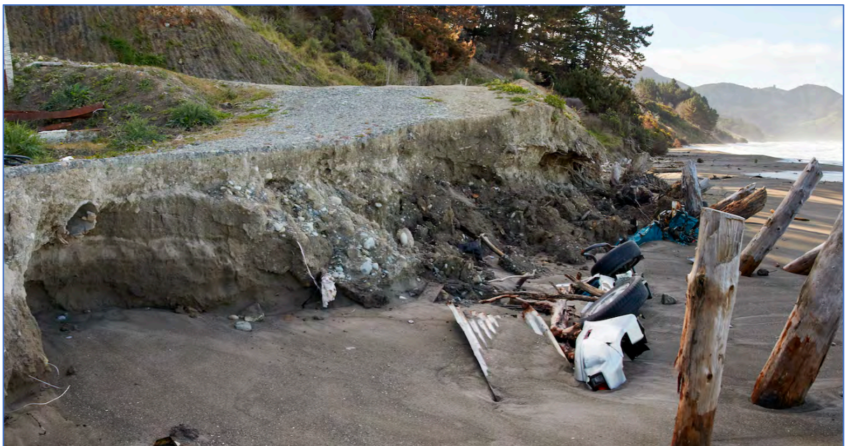
Figure Sixty Four. The road heading up to the last property at the end of McIlroy Road showing the scour and undercutting associated with the broken culvert, the car bodies and other debris used as armouring on the fill making up the access track and the “totem poles” used to buttress the slope. Note the over steepened face and overhangs.
