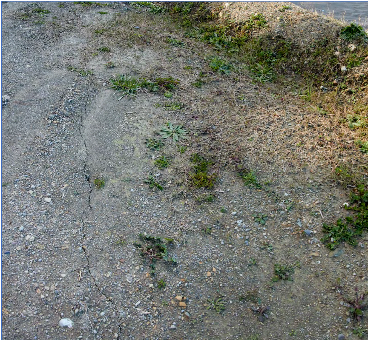
Figure Sixty Five. Tension cracks on the bend in the road leading up to the last house.
