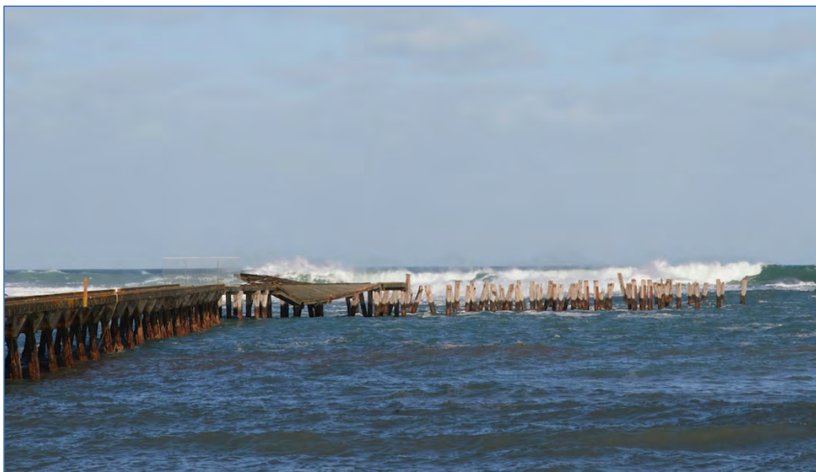
Figure Sixty Six. Additional damage to the Tokomaru Bay wharf as a result of heavy seas
