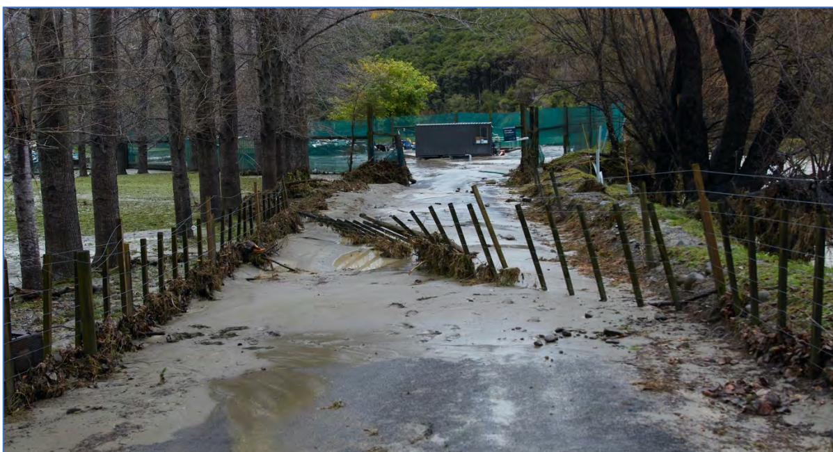
Figure Fifty. Flood impacts at the Tokomaru Transfer Station.
