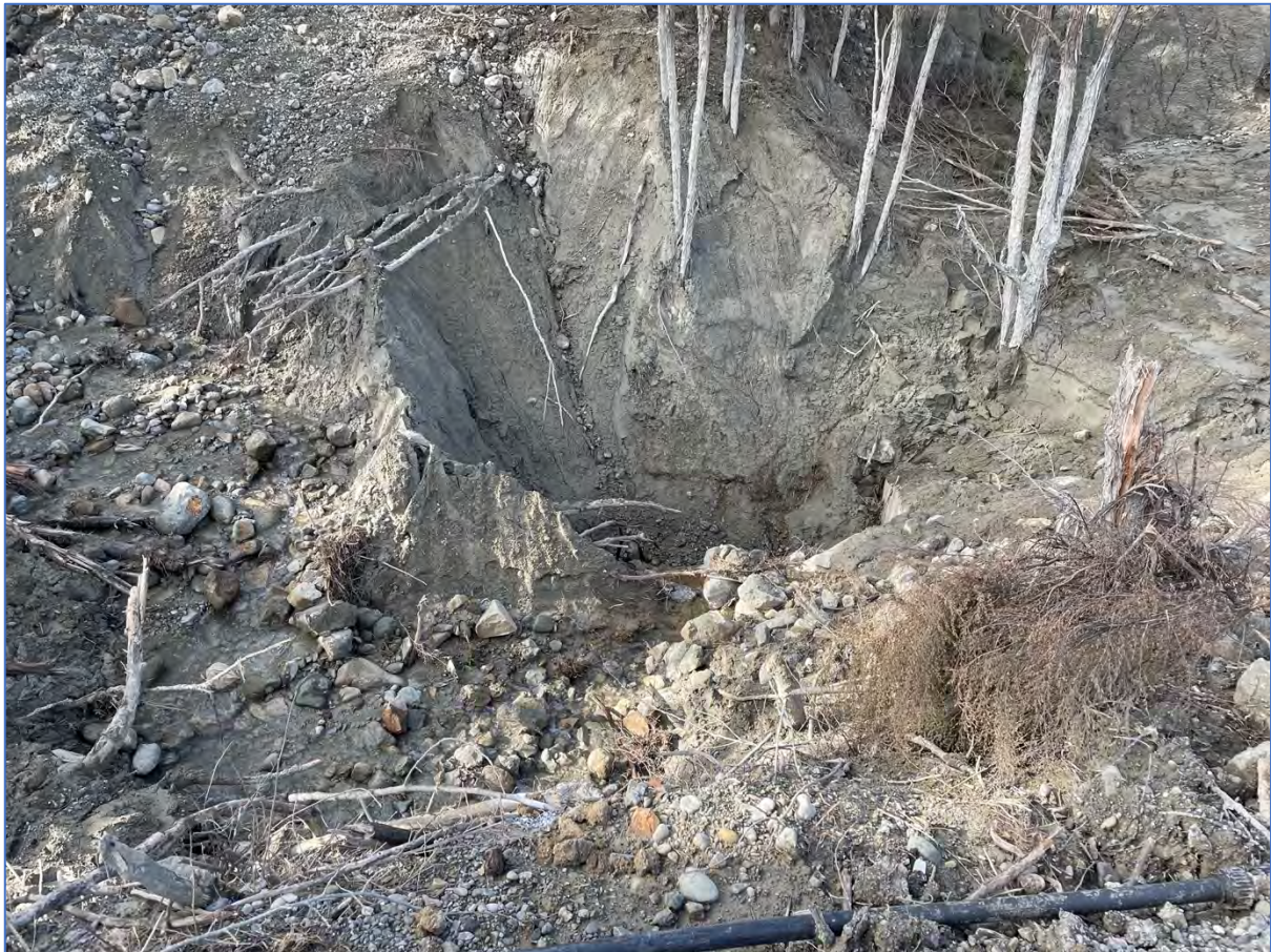
Figure Fifty Four. View of culvert on State Highway 35 north of Tokomaru Bay after clearing. This shows that only a small pit has been dug at the inlet to allow for drainage. It is understood that further clearance is planned and that an assessment is underway to increase culvert capacity.
