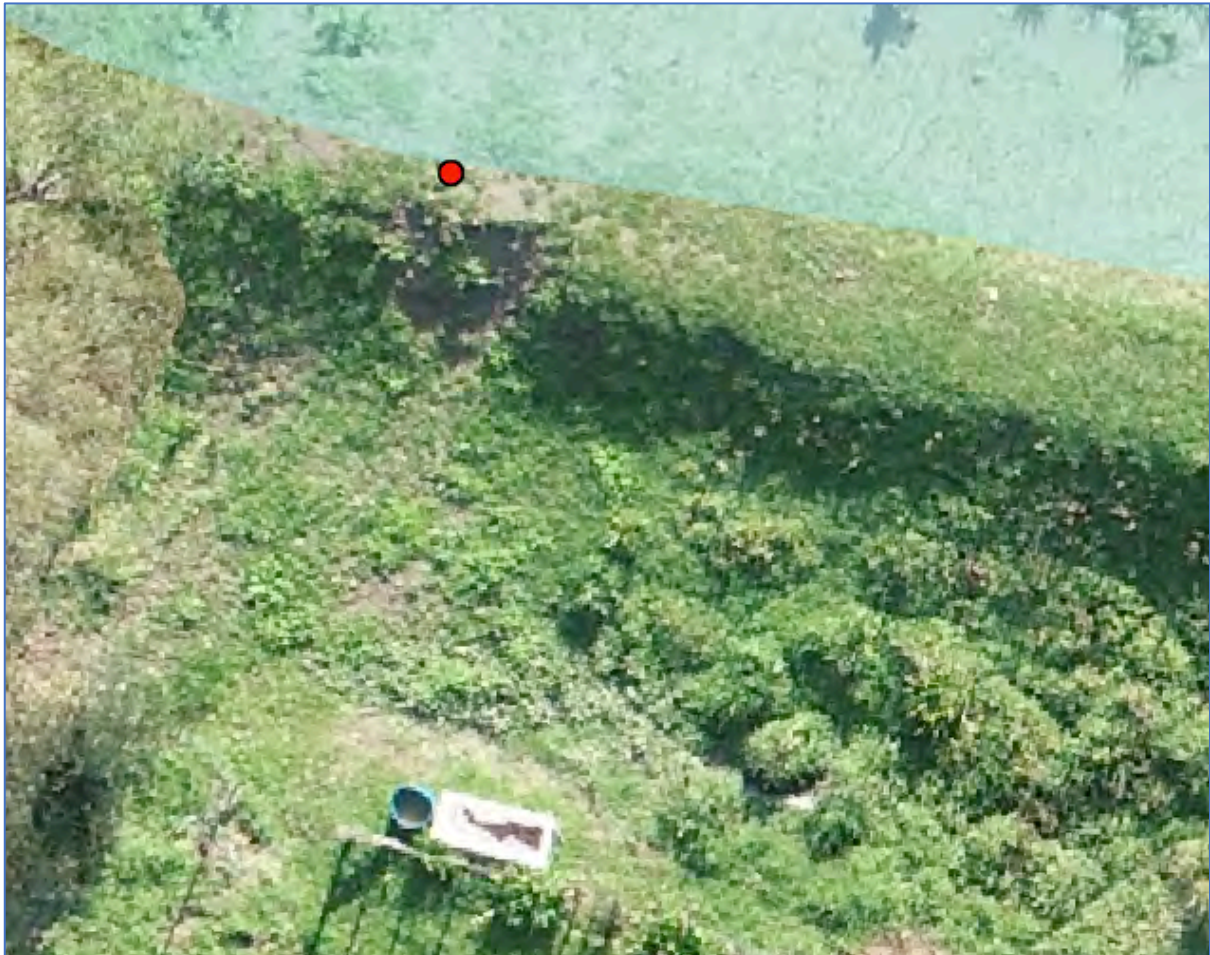
Figure Fifty Seven. View of the upper overtopping point showing the silt deposition and the indications of stopbank erosion.
