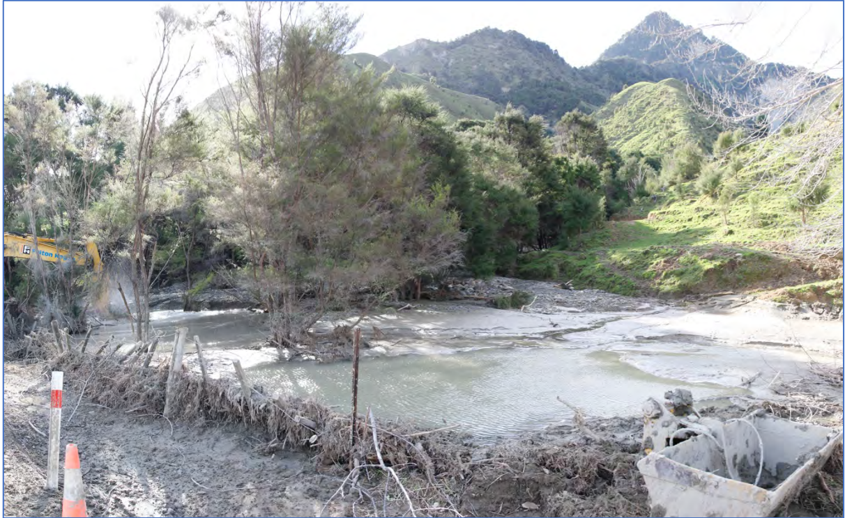
Figure Fifty Two. View of culvert on State Highway 35 north of Tokomaru Bay prior to clearing. Note the extensive infill of debris and the indications of overtopping on the fenceline.
