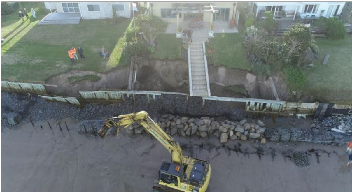
DAMAGE TO SEAWALL ACROSS 22-26 PARE STREET (source: GDC resource consent application)
