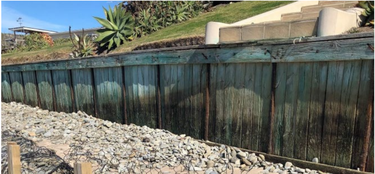
TYPICAL VIEW OF RETAINING WALL ON NUMBERS 24 & 26 PARE STREET (PRIOR TO 2019 STORM EVENT)
