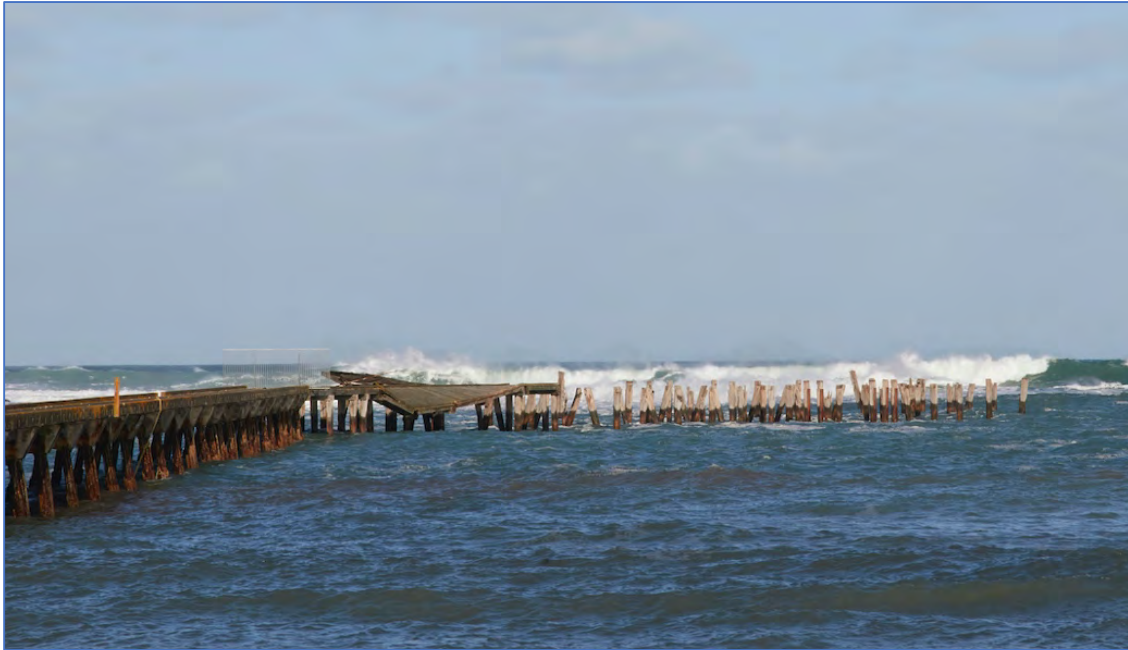
Figure Sixty Six. Additional damage to the Tokomaru Bay wharf as a result of heavy seas
