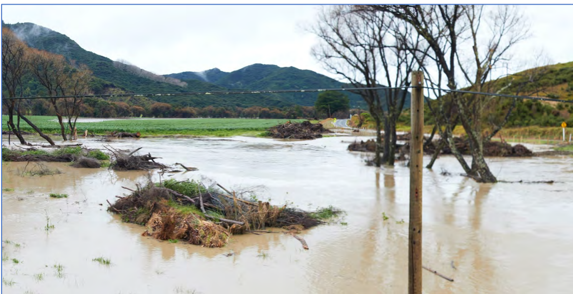
Figure Eleven. Willow piles being eroded upstream of State Highway 35 Bridge, Mahanga Stream.
