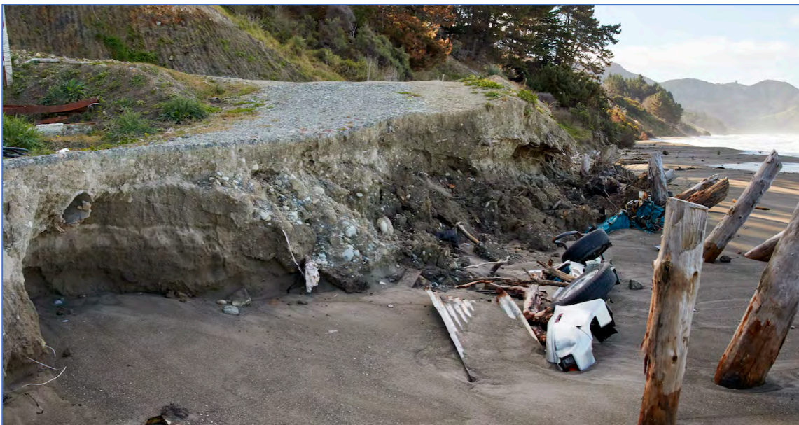
Figure Sixty Four. The road heading up to the last property at the end of McIlroy Road showing the scour and undercutting associated with the broken culvert, the car bodies and other debris used as armoring on the fill making up the access track and the “totem poles” used to buttress the slope. Note the over steepened face and overhangs.
