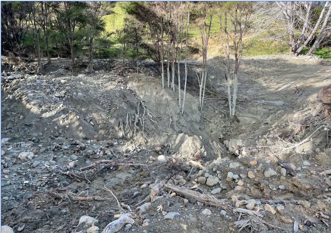
Figure Fifty Three. View of culvert on State Highway 35 north of Tokomaru Bay after clearing showing the considerable volume of debris remaining above the inlet.
