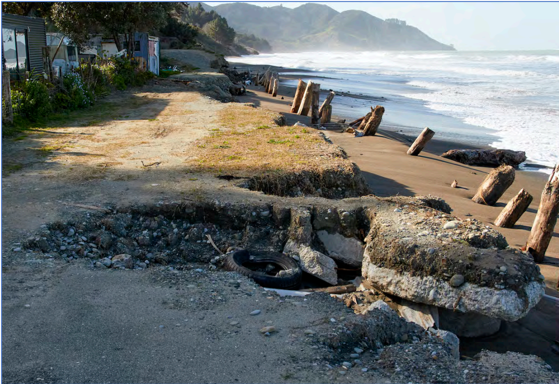
Figure Sixty Three. The extent of scouring and channelling of the road.
