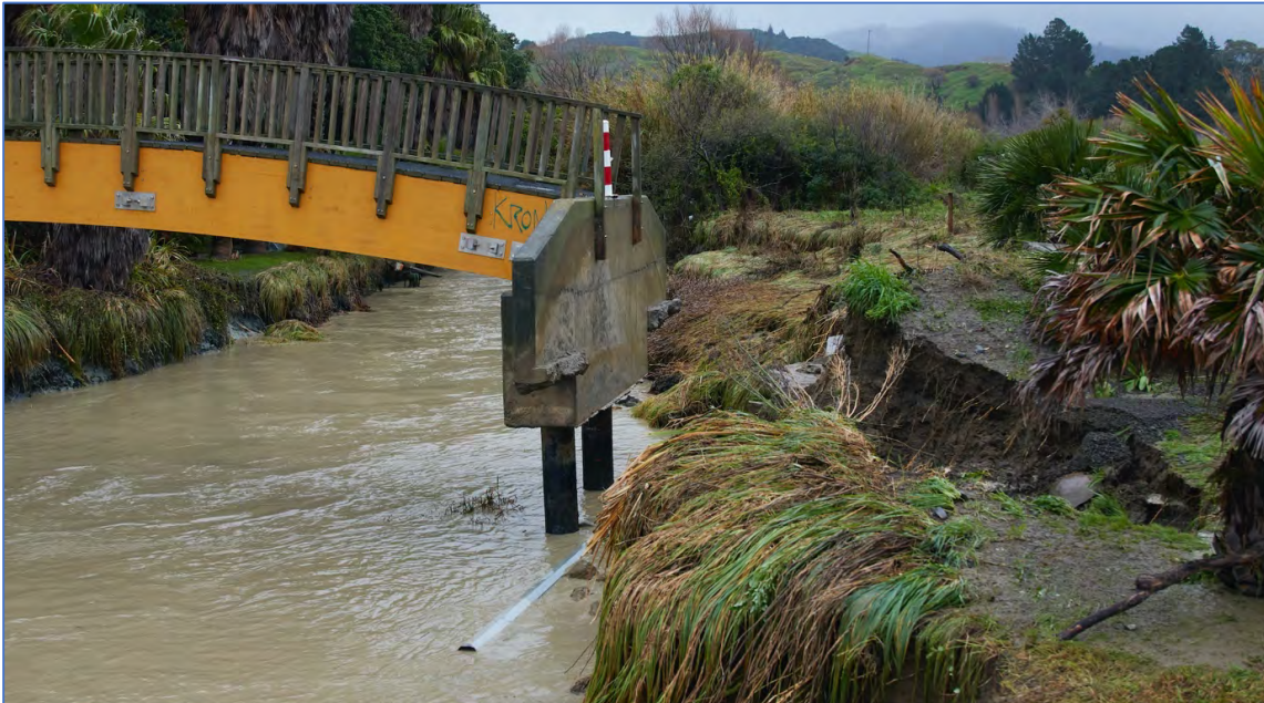
Figure Forty Nine. The washed out abutment of the footbridge at the mouth of Waiotu Stream.
