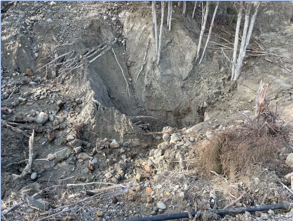
Figure Fifty Four. View of culvert on State Highway 35 north of Tokomaru Bay after clearing. This shows that only a small pit has been dug at the inlet to allow for drainage. It is understood that further clearance is planned and that an assessment is underway to increase culvert capacity.
