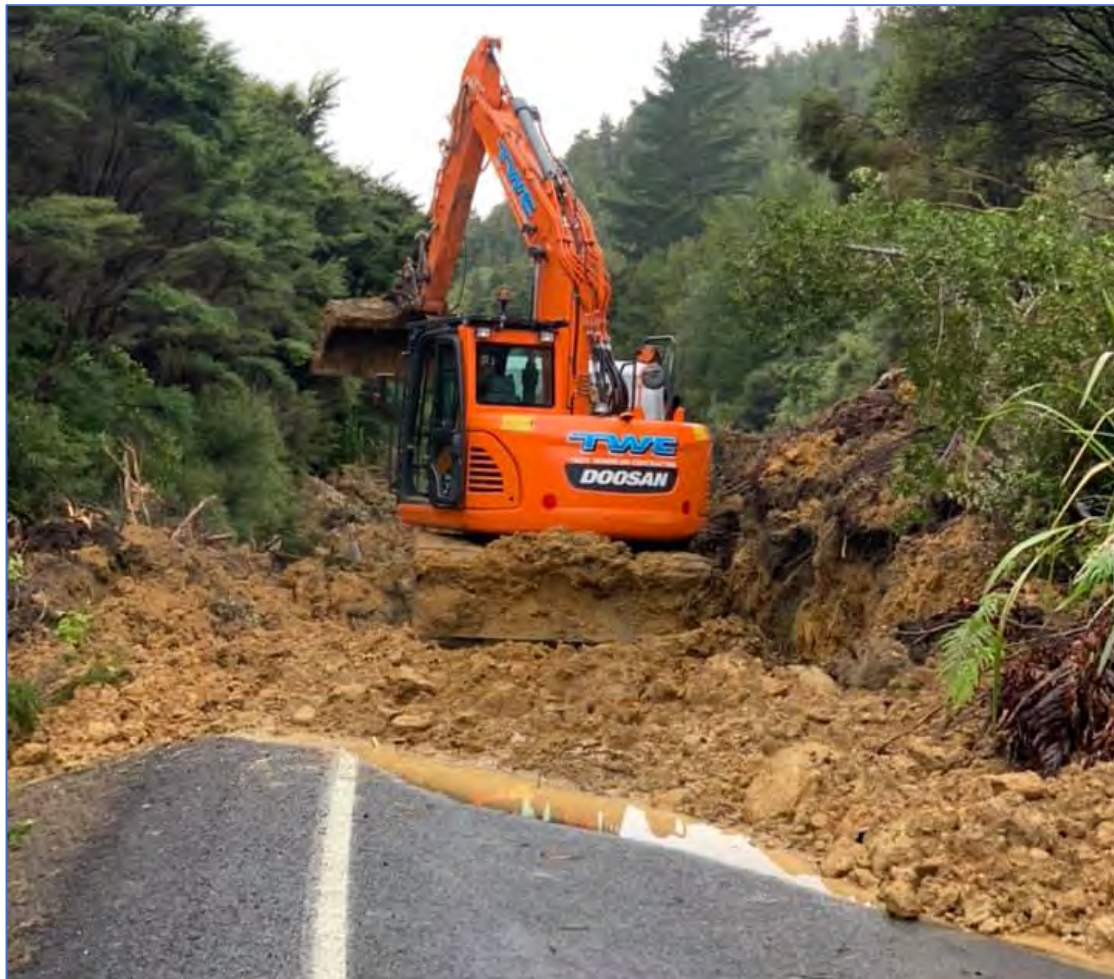
Figure Six. Clearing the significant slip blocking State Highway 35 at Oweka close to the Lottin Point turn off (photograph Rex Rongo Stainton).
