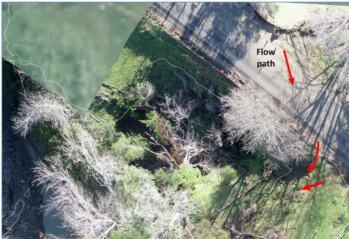
Figure Fifty One. drone footage of the blocked culvert on State Highway 35 showing the overland flow path to the creek downstream of the culvert.
