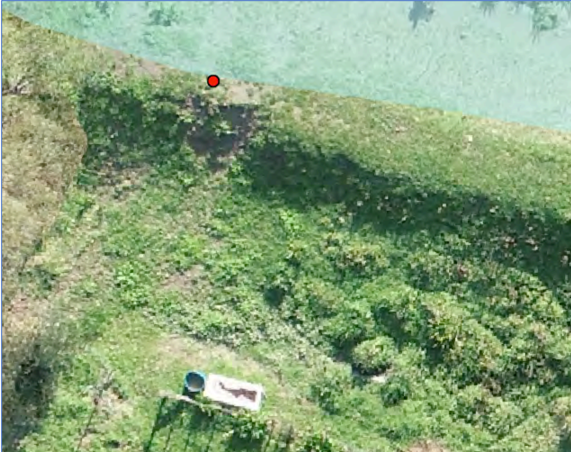
Figure Fifty Seven. View of the upper overtopping point showing the silt deposition and the indications of stopbank erosion.
