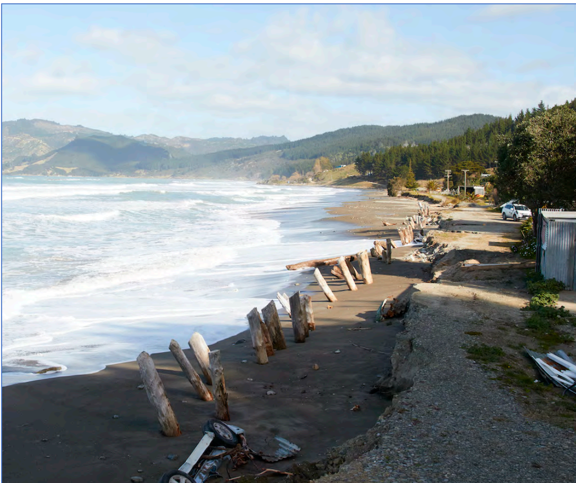
Figure Sixty Two. The extent of recent coastal erosion at the northern end of McIlroy Road marked by the pine logs that had been pushed into the sand as retaining posts.
