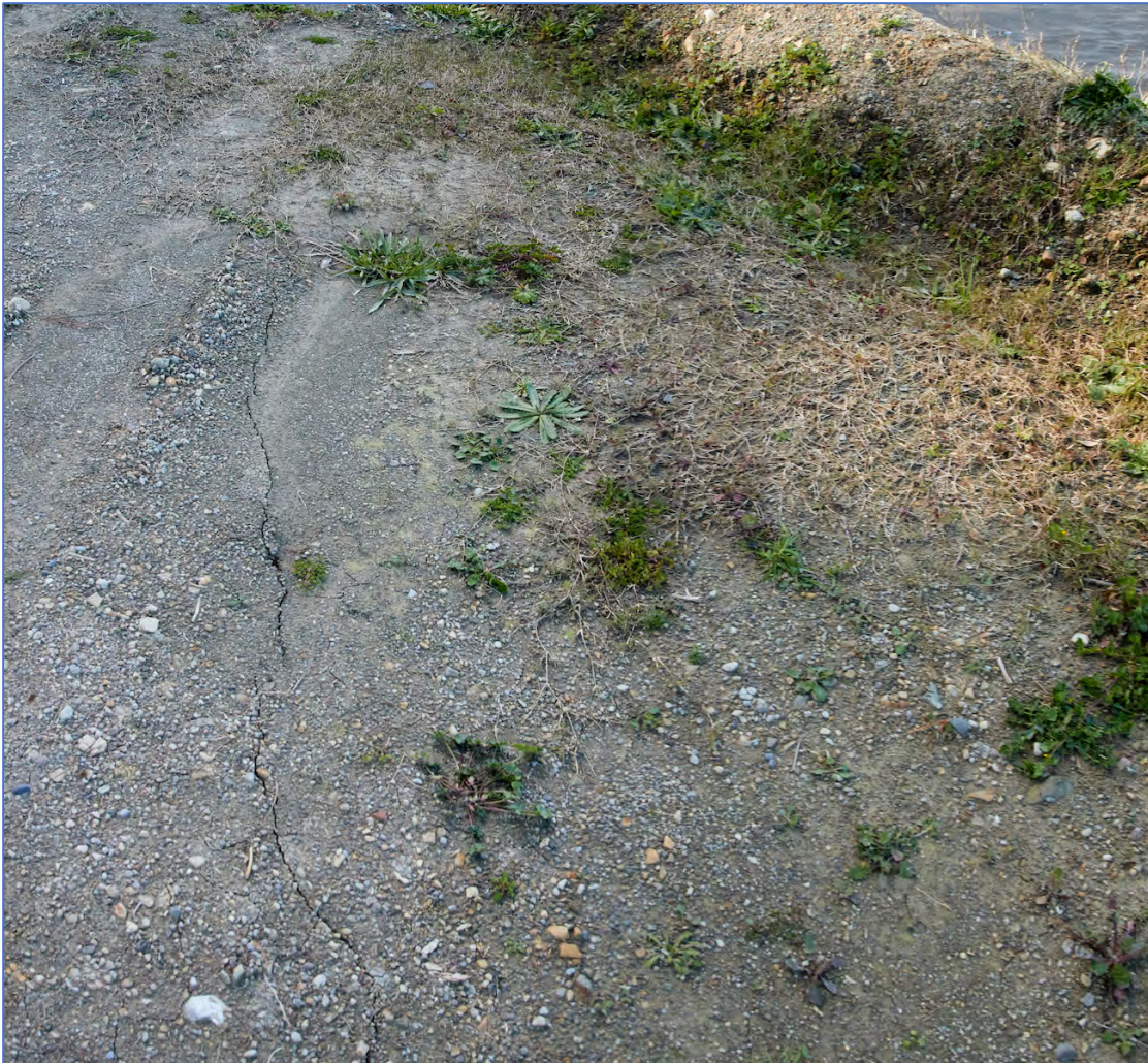
Figure Sixty Five. Tension cracks on the bend in the road leading up to the last house.
