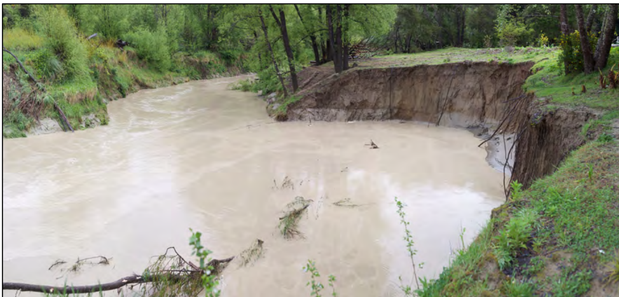
Figure Twelve. View of the logjam site and eroded embayment on the 15 th October (refer to Figure Three for the state of the embayment prior to the 15 th -16 th October). While the relative lack of turbulence may have indicated that the logjam had flushed out, the evidence was not conclusive.
