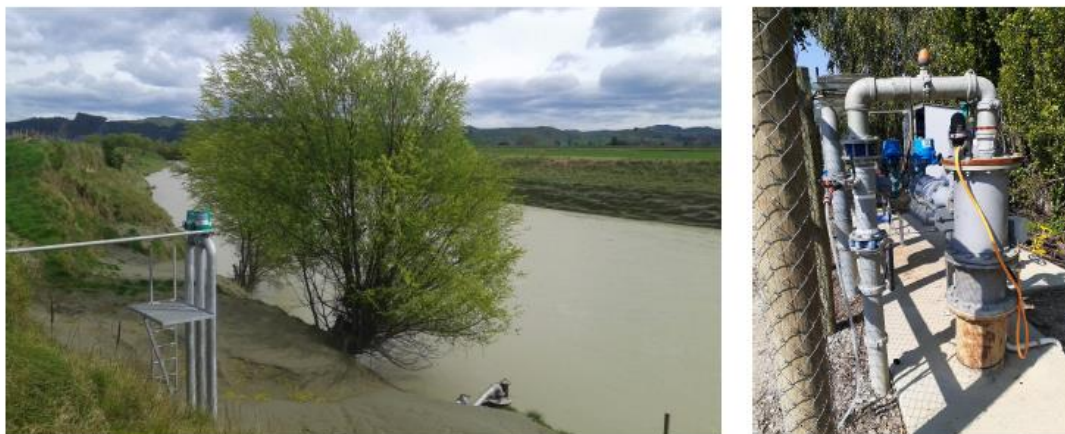
Figure 4: Managed Aquifer Recharge - Waipaoa River intake on the left and MAR injection bore on the right
