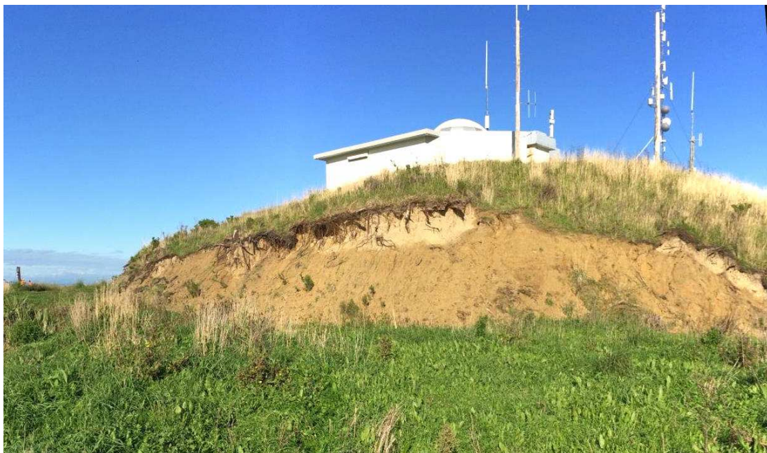
Figure 11: Eastern cut slope in May 2017 showing cut face affected by erosion and shallow seated landslippage since original earthworks.
