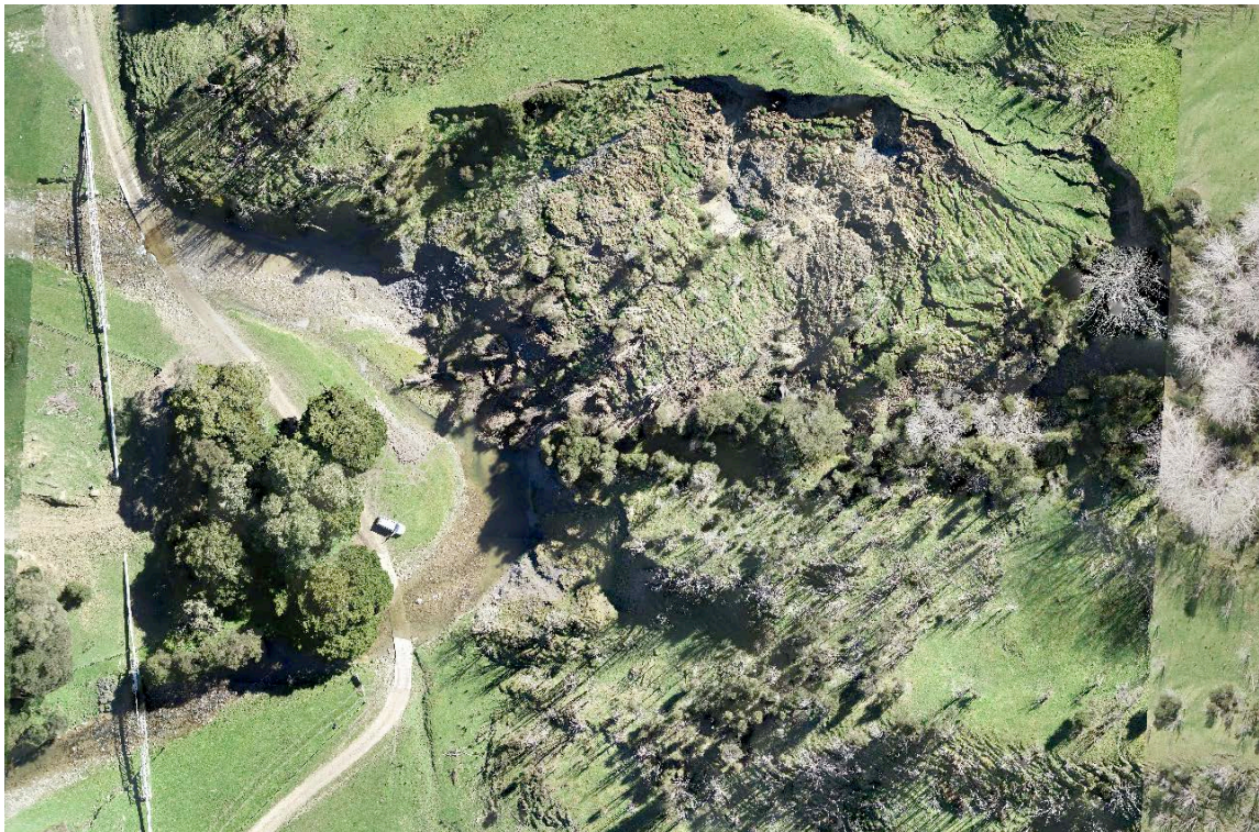
Figure Five. Drone map of the landslide from 29 th September 2021. Vehicle middle left gives scale. The flight was taken after emergency works were completed to divert the river away from the toe of the landslide into the flood channel. The pipeline is 58 to 62m away from the toe of the landslide at the end of September.
