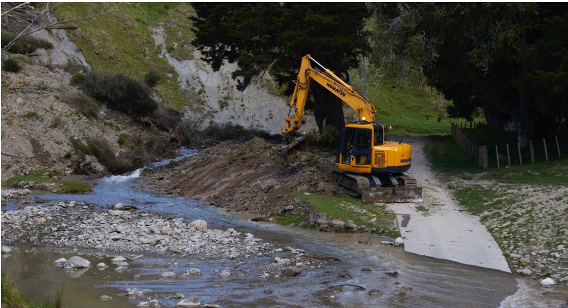
Figure Nine. Fulton Hogan undertaking channel reinstatement under emergency works. It needs to be noted that Fulton Hogan assigned their best digger operator to the works and as a result sediment discharge downstream was limited.
