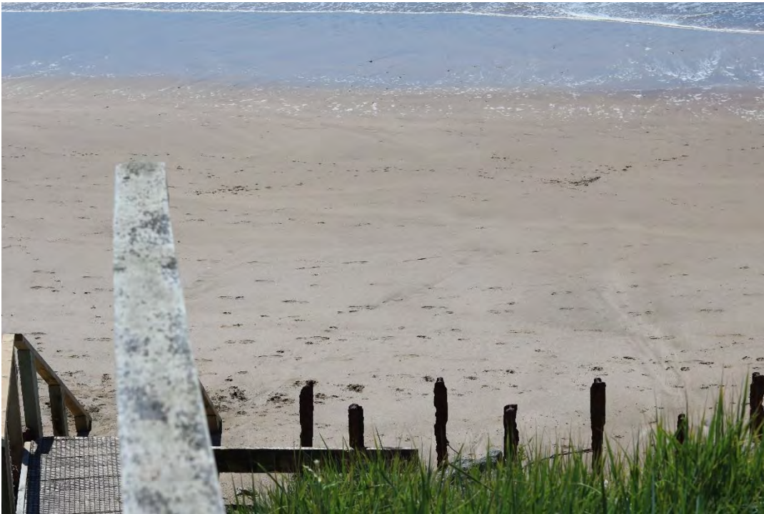
Figure 11: Photo from Viewpoint 4, midway down the public stair access looking south along the rock revetment site. A3 size version of the viewpoint is provided in Appendix D .
