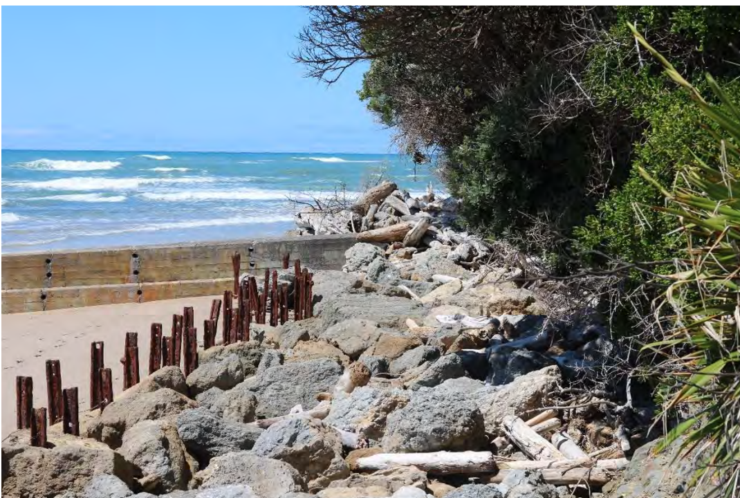
Figure 12: Photo from Viewpoint 5, midway down the public stair access looking south along the rock revetment site. A3 size version of the viewpoint is provided in Appendix D .
