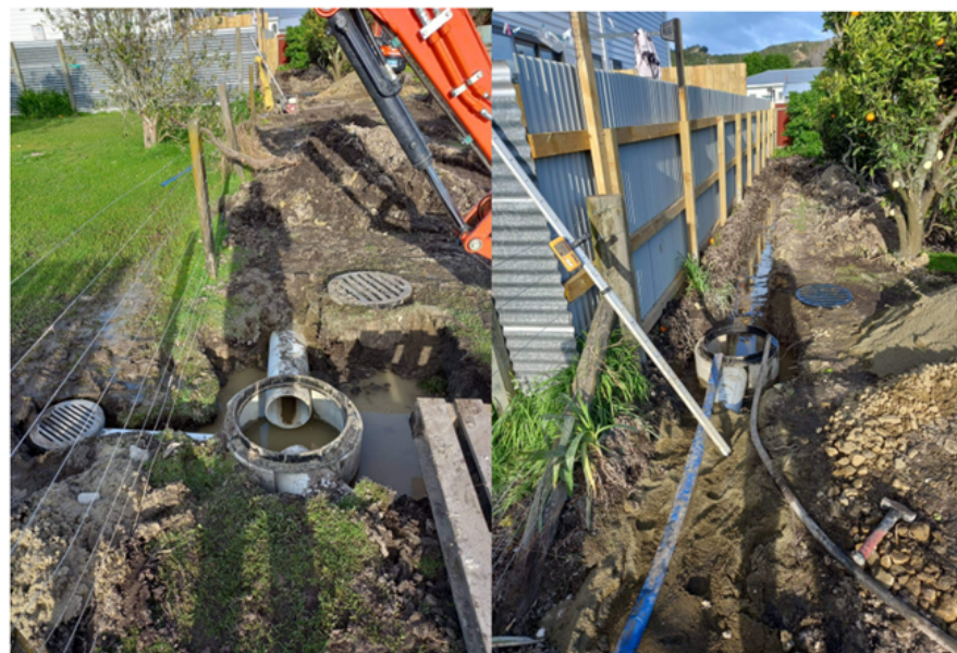
Additional bedding of 65mm basecourse was placed in trenches due to soft underground services
