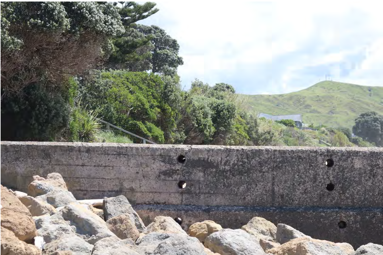
Figure 9: View from the south side of the groyne, along the edge of the protective rock revetment in this area.
