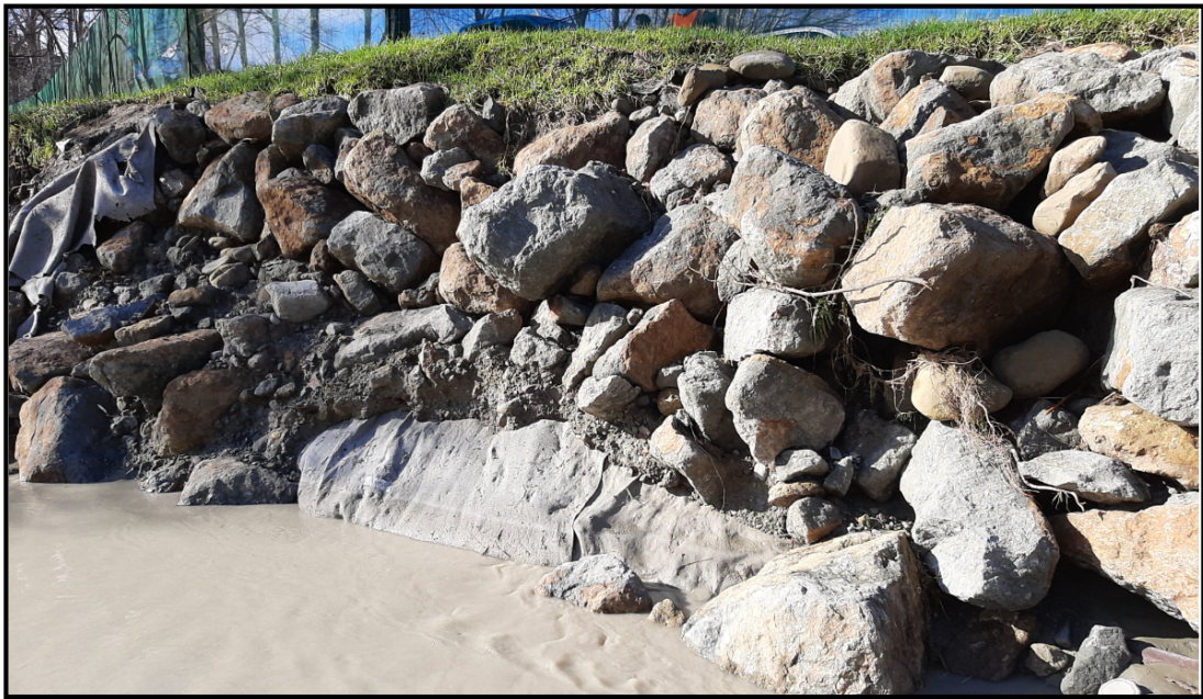
Figure 4, damage to Revetment wall
