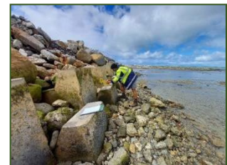
Fig 22: Eruera Ria from Ecoworks NZ measures the front face of the akmon toe blocks at low tide.
