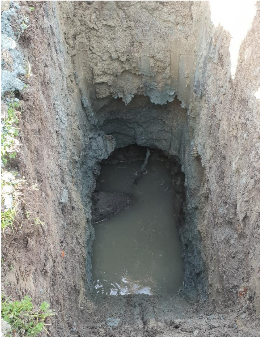
Photograph 5: TP07, water accumulation at 3.0 m bgl.
