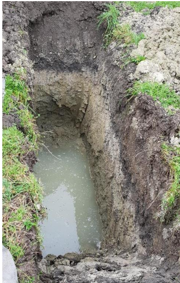
Photograph 2: TPO5 - water seepage and accumulation at 1.9m bgl.
