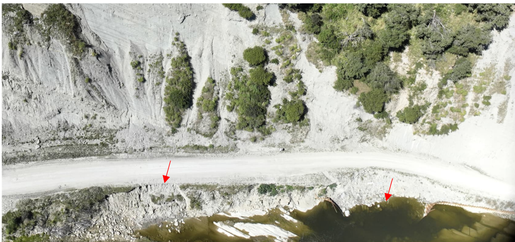
Figure 4: Mid to western extent of Bluff 1, showing with arrows areas where road width has been affected by a drop-out and the compromised sheet pile wall.
