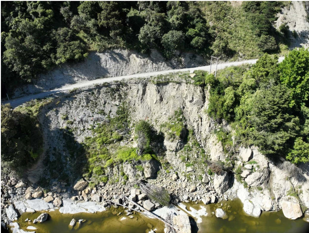
Figure 12: View to southwest of large underslip narrowing the roadway beneath Bluff 3. Contractors have cut back into the slope toe to widen the road, exposing highly weathered weak rock.
